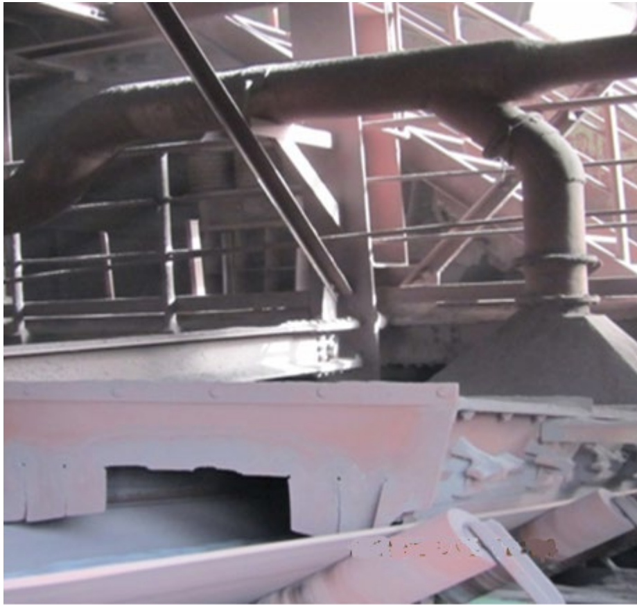
Figure 4. Inappropriate connection of branching down
